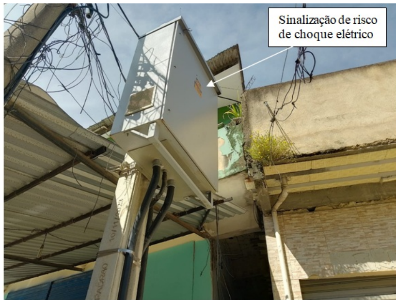
Foto 11 – Cabine do painel
