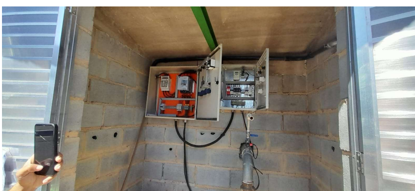
Painel Elétrico Soft starter, CCO
