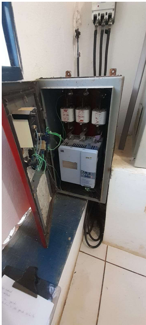
Chave Soft start Motobomba 4
