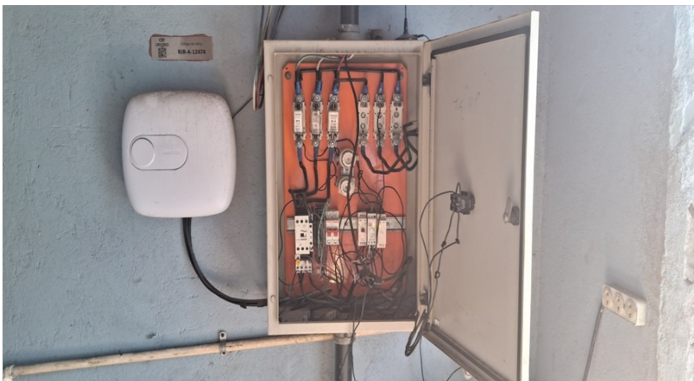
Foto 4 – Paineel de controle.
