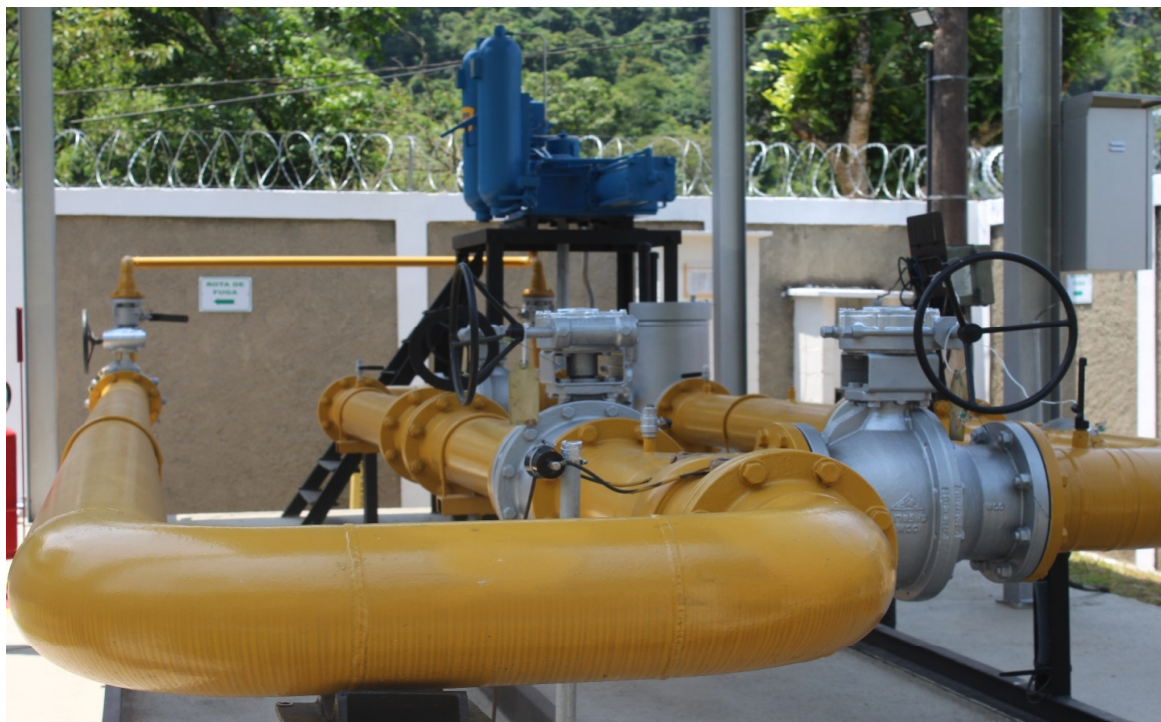
Foto 7: By pass e válvulas
